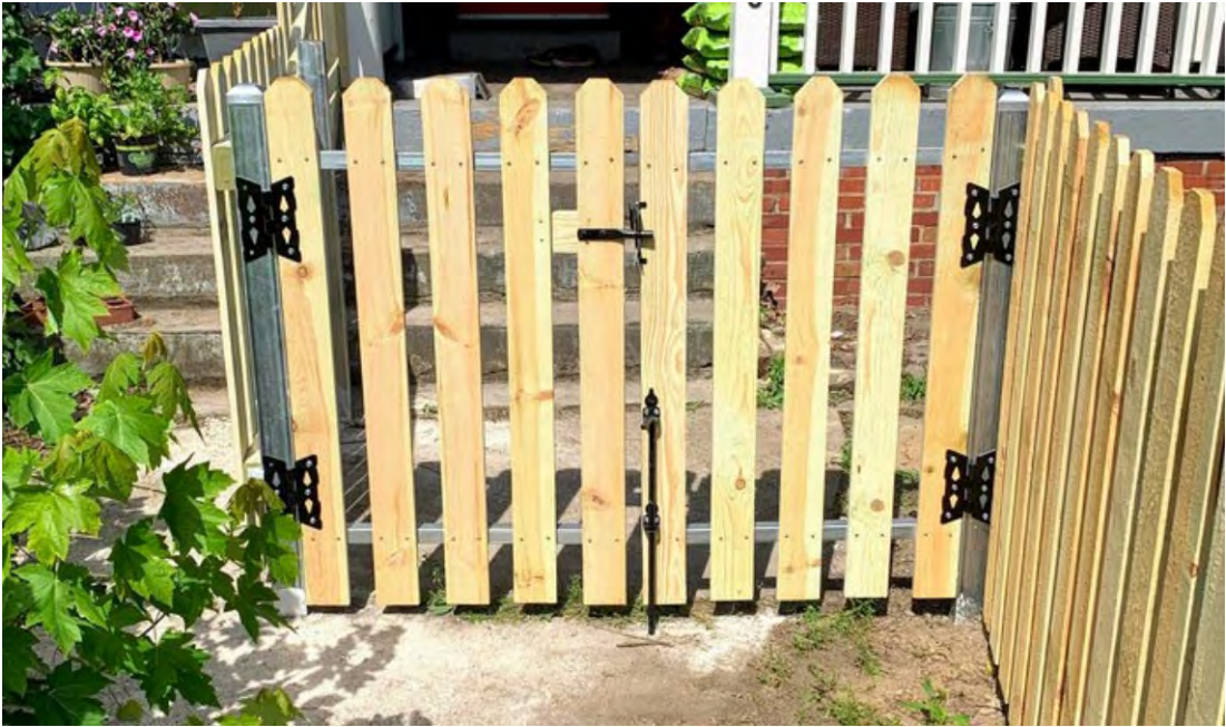
Figure 5. Example of gate to be installed - 8' wide double gate, to swing inward only
