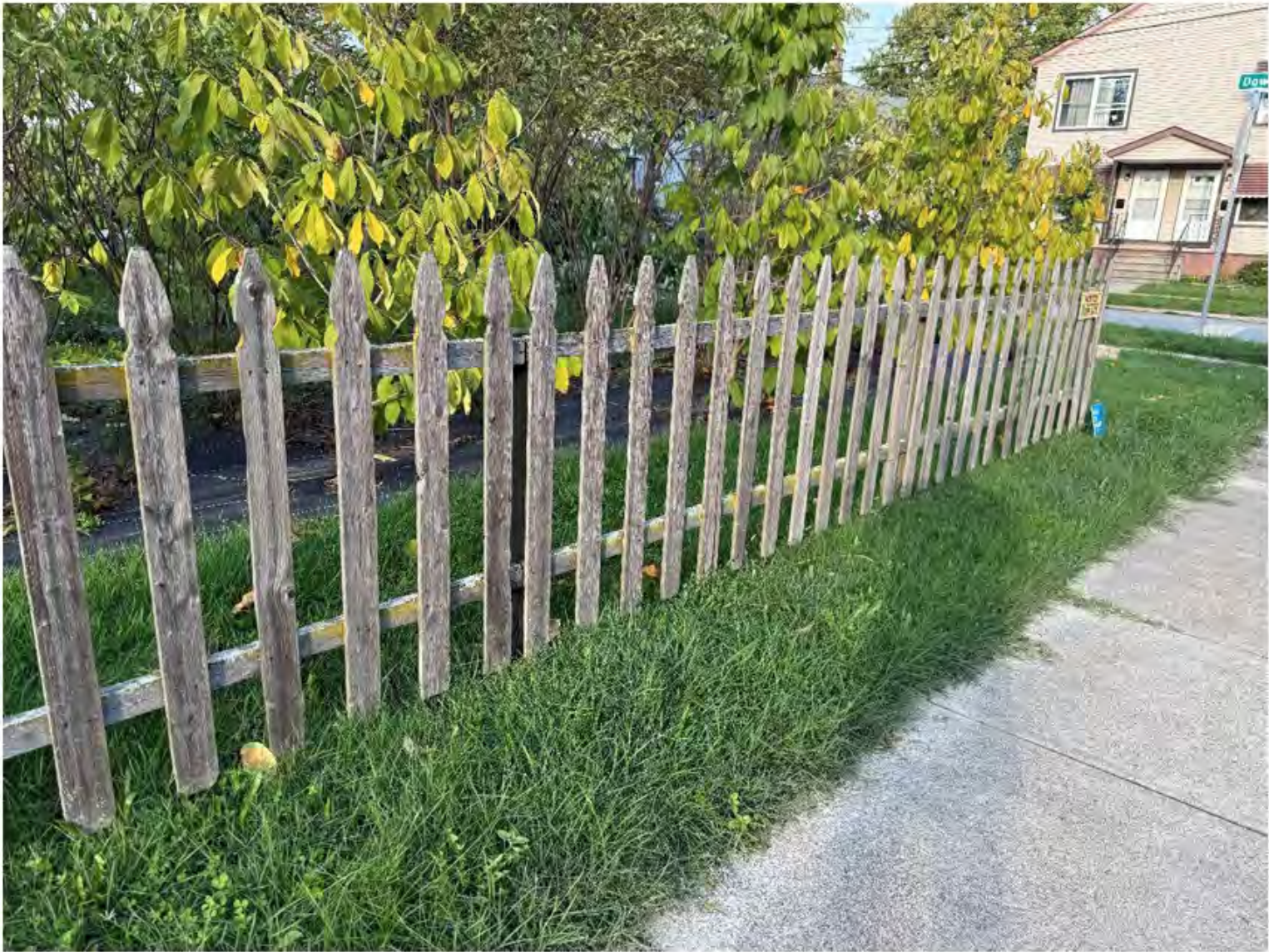
Figure 2. View of current fencing (to be removed and replaced) near intersection of Dowd and Thrush.
