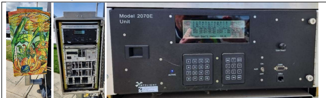
Figure 8 – Madison Ave & Hilliard Rd/Carabel Ave (2070 controller Unit)
